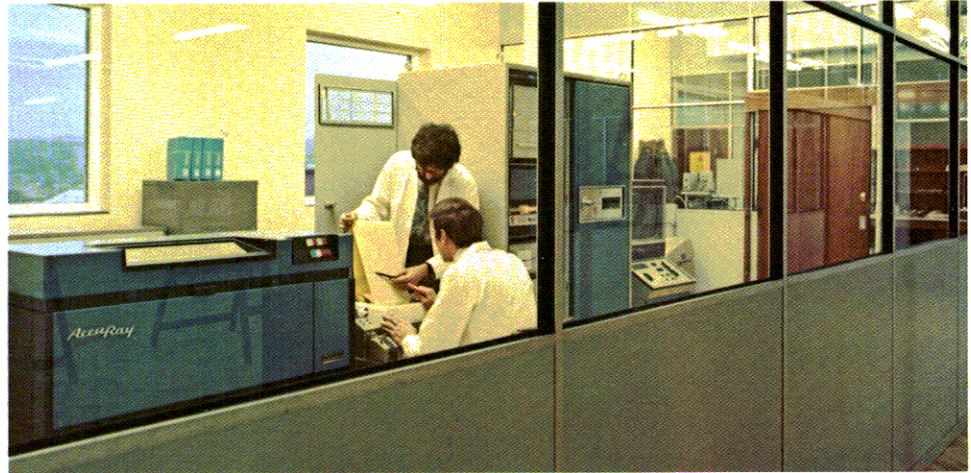
AccuRay 1000 central computer room in this United Kingdom cigarette plant is source of comprehensive production and quality data for management.
