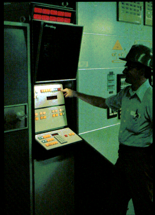
AccuRay system displays key process variables for operating personnel in central control room.
