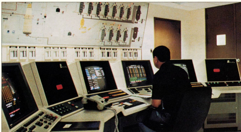
With more computer-to-computer communications capabilities than any other process control supplier, AccuRay systems such as this pulp mill system can effectively manage other computers to control complex processes.
